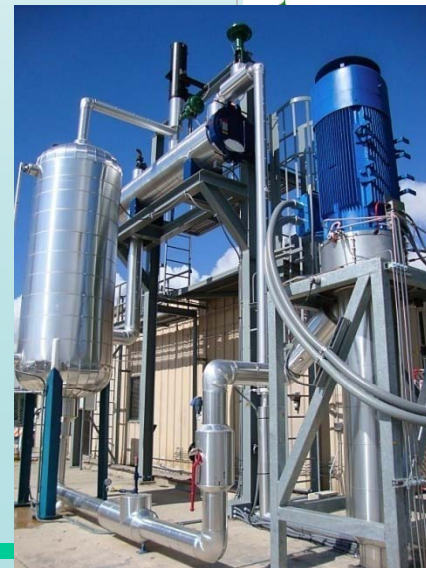
Liquid CO 2 Pump Loop
