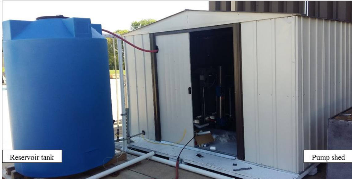
Figure 28. Reservoir tank (left) and pump shed (right) accommodating two pumps and heat exchanger located outside of test-cell.
